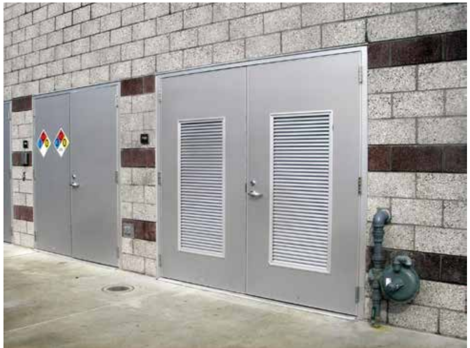
Aluminum flush doors (closed-cell foam injected) with aluminum louvers on a chemical storage room.
