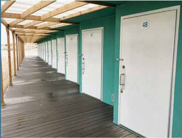
Pultruded fiberglass doors (closed cell foam core) at beach cabanas at Lido Beach on the New York coast.
