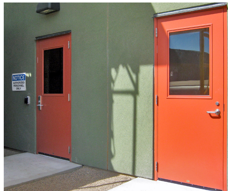
Aluminum Flush Doors (SL-16) with painted finish - Ina Road Water Reclamation Facility in Tucson, AZ
