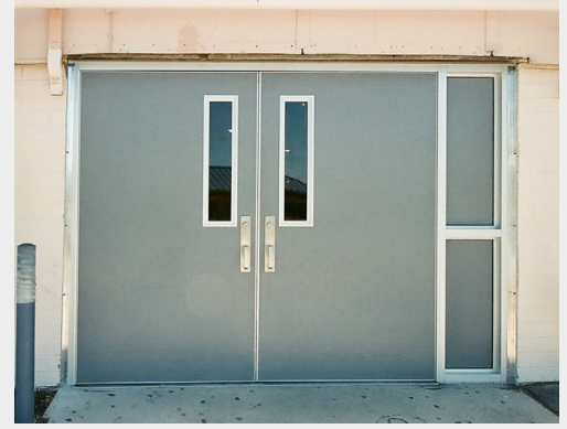
AFTER: Special-Lite Door System installed in the “worst” entrance of the school demonstrates durability. Doors now operate trouble-free and resist forced entry attempts.
