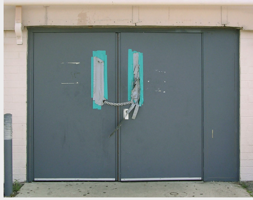
BEFORE: Integral locks become deformed due to excessive pulling on the door, leading the maintenance department to chain the doors shut to counter repeated break-ins.
