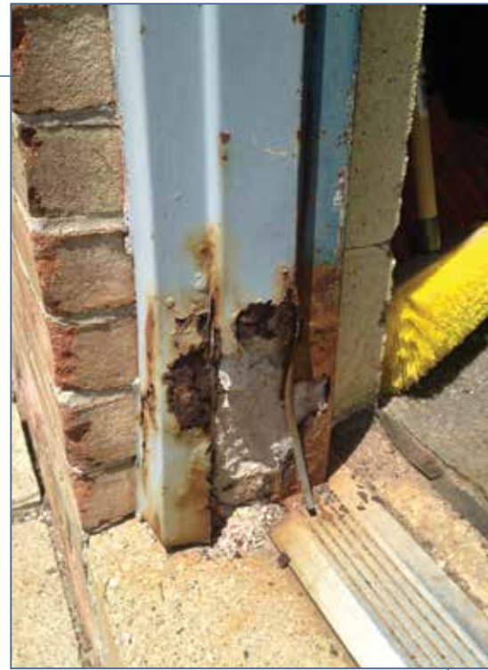
Example of hollow metal frame rusted and corroded from the elements
